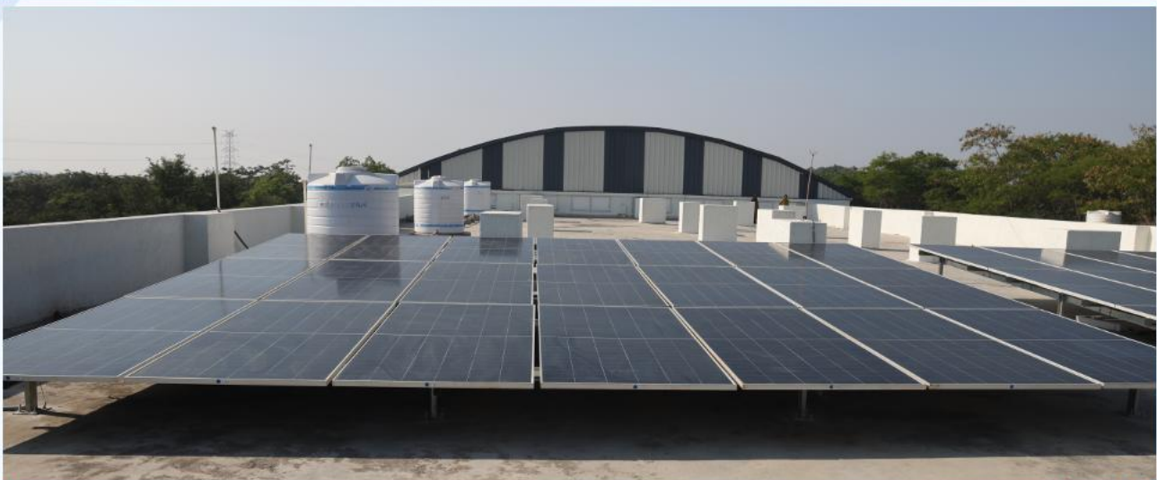
Newly Commissioned Solar Power Plant (50 KW p ) installed at Kreedha Bhavan, TGPA
